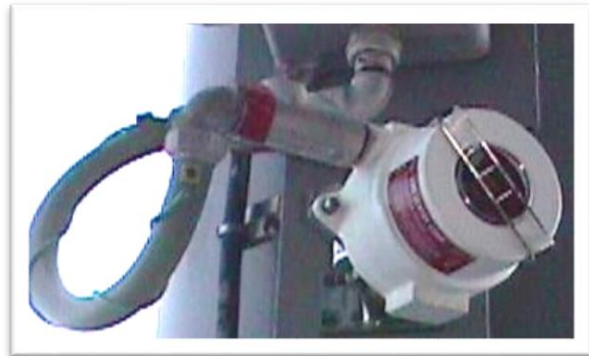
Above: Honeywell SS4 Flame Detector installed with explosion-proof conduit seal at conduit entry point.
